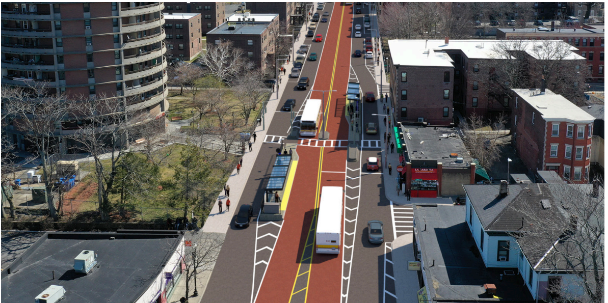
Columbus Avenue dedicated bus lanes, under construction in early 2021. Source: Massachusetts Department of Transportation (MassDOT)
