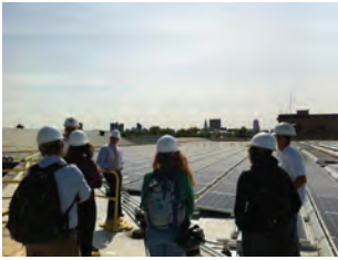
In May 2012 Harvard Athletics completed a six week renewable project as it installed a layer of 2,275 solar panels on the roof of Gordon Track. Harvard now has over 1MW of installed solar capacity from on campus projects.
