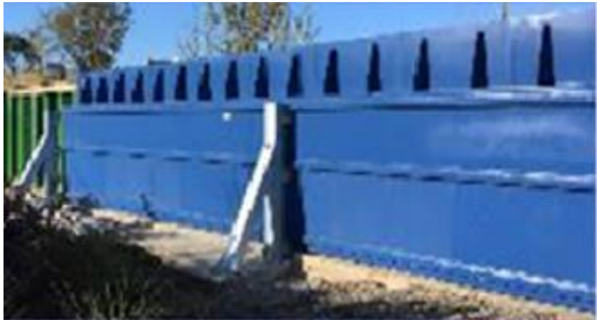
SLIDING FLOOD GATES
