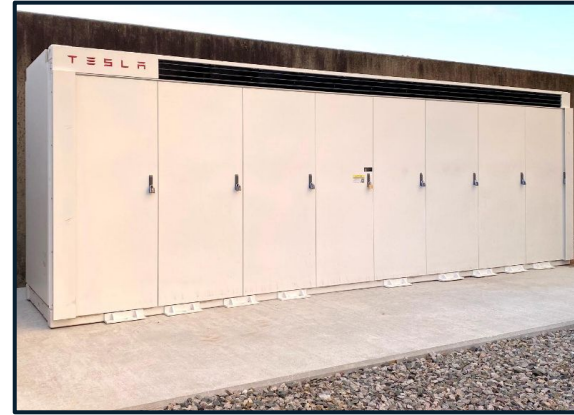
~575 kW BESS - Boston, MA
