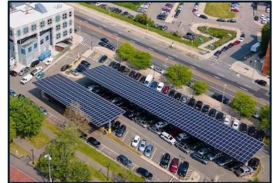
250 kW Solar Canopy - Roxbury, MA
