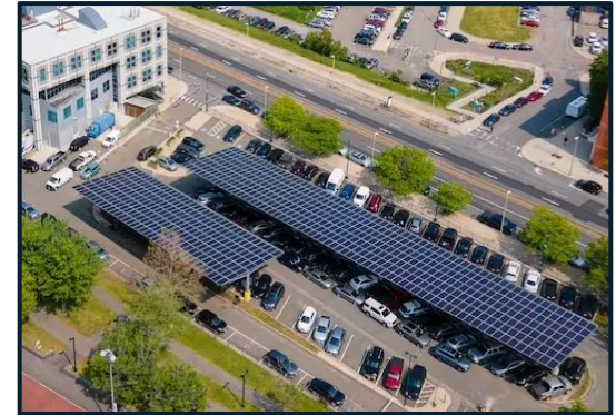
250 kW Solar Canopy - Roxbury, MA
