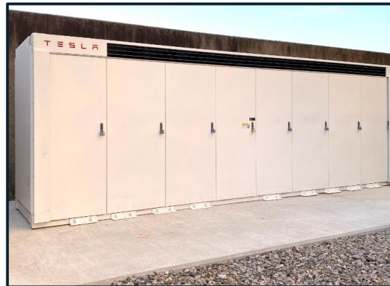
~575 kW BESS - Boston, MA
