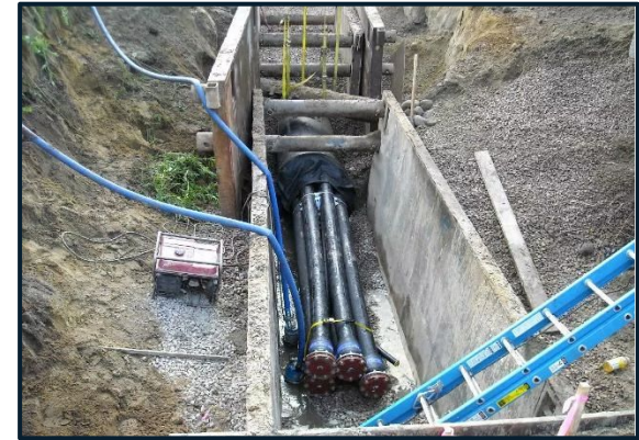
Underground Electric Transmission Lines
