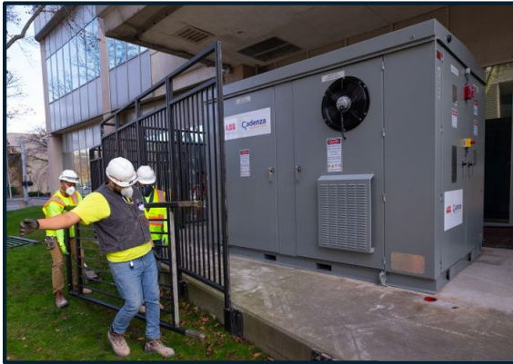
250 kWh BESS - Westchester, NY
