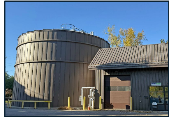
300 kW Anaerobic Digester - So. Burlington, VT
