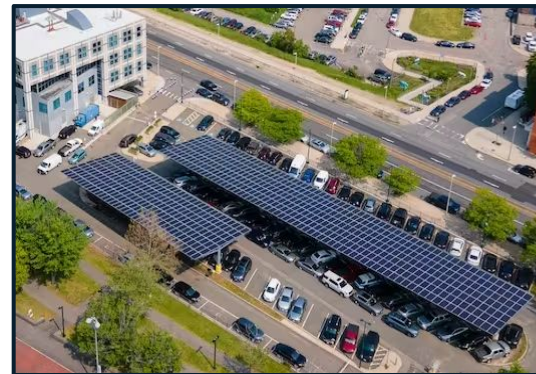
250 kW Solar Canopy - Roxbury, MA
