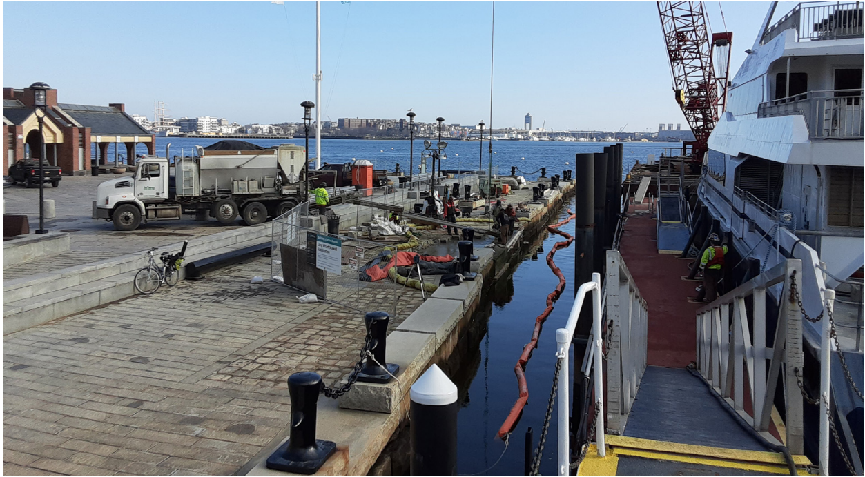
The Long Wharf Seawall Stabilization project is expected to be completed in early 2021.
